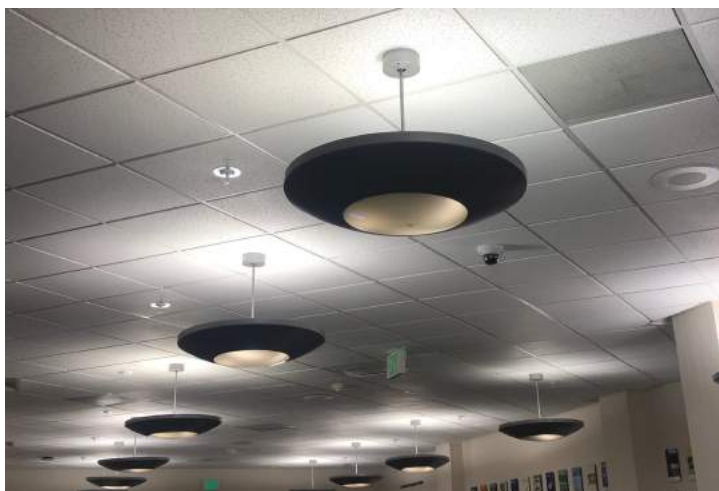
Figure 4.16: Acoustic ceiling tiles example.
